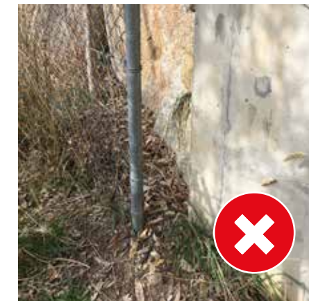
Gap between chainlink fencing & culvert wing wall
