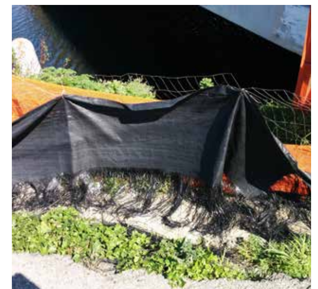
Wire mesh, silt fencing & orange plastic mesh deteriorating on site boundary, USA
