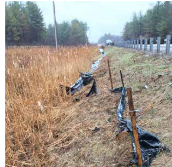
Silt fencing obliterated after vegetation clearance along a roadside in Canada
